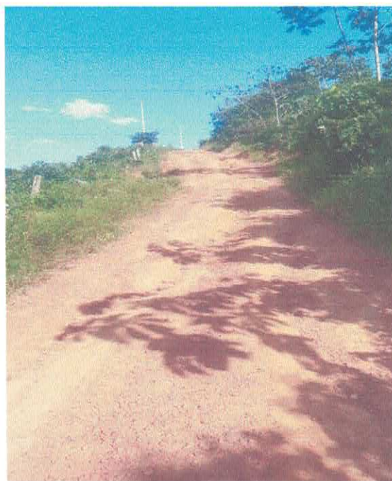
Trecho critico km 9,0 Vic 15
